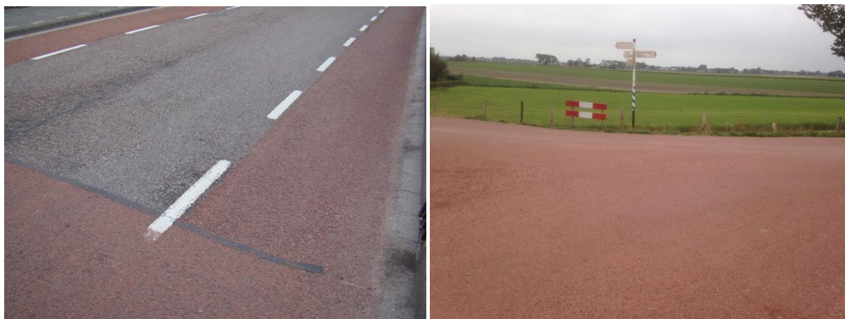
Figure 5 and 6: Typical damage pattern of red asphalt with unmodified clear binder. Date of construction for the situation on the left was around 2004. Ravelling was clearly visible here in 2019, but this also applied to the intermediate (black) asphalt.
