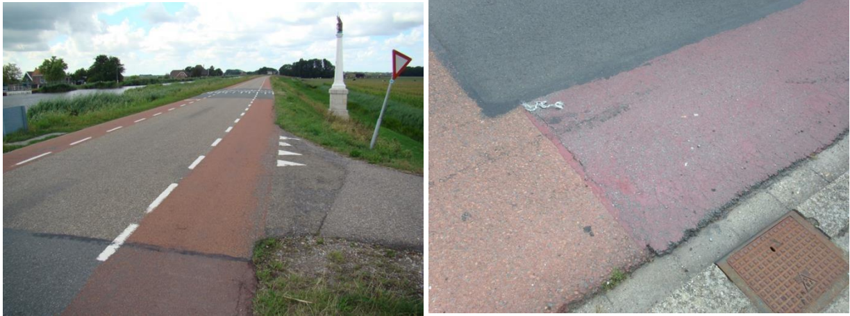
Figure 1: Left bituminous surface treatment.
