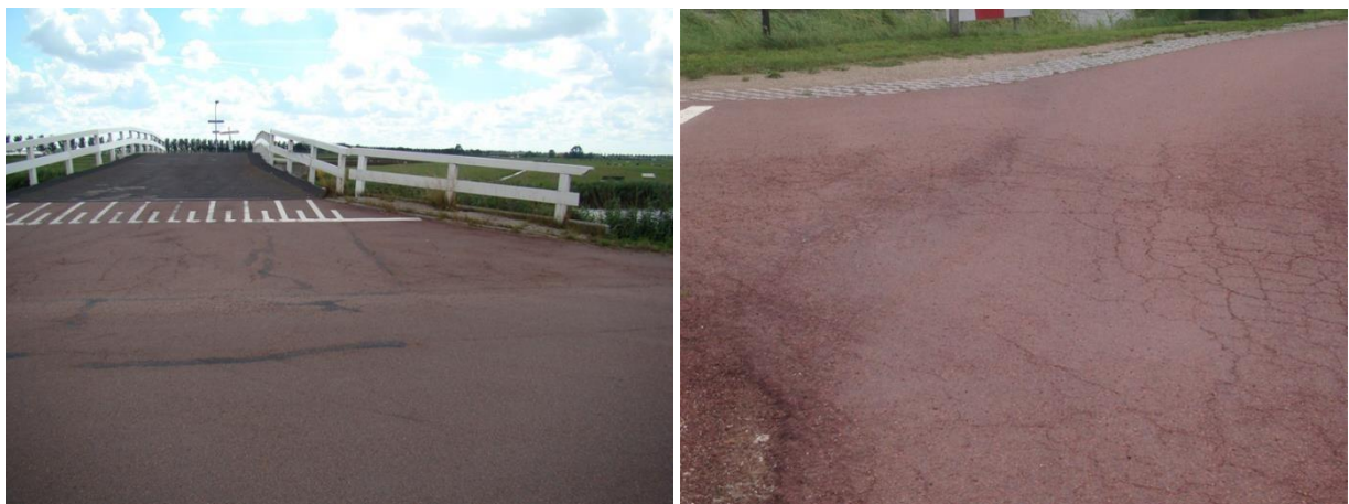
Figure 3 and 4: Typical damage pattern of red asphalt with black bitumen. Exact date of construction is not known, but probably less than 10 years ago.
