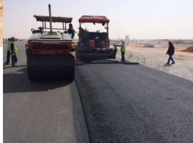
Construction of New aprons to the East of the Commercial Galleries at King Khaled International Airport
